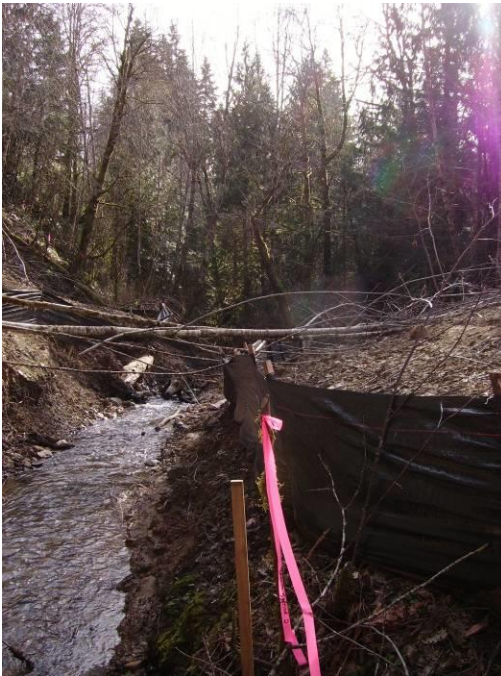
(Post-Project) Looking downstream at stream channel Following removal of stream crossing (road fills and culverts).
