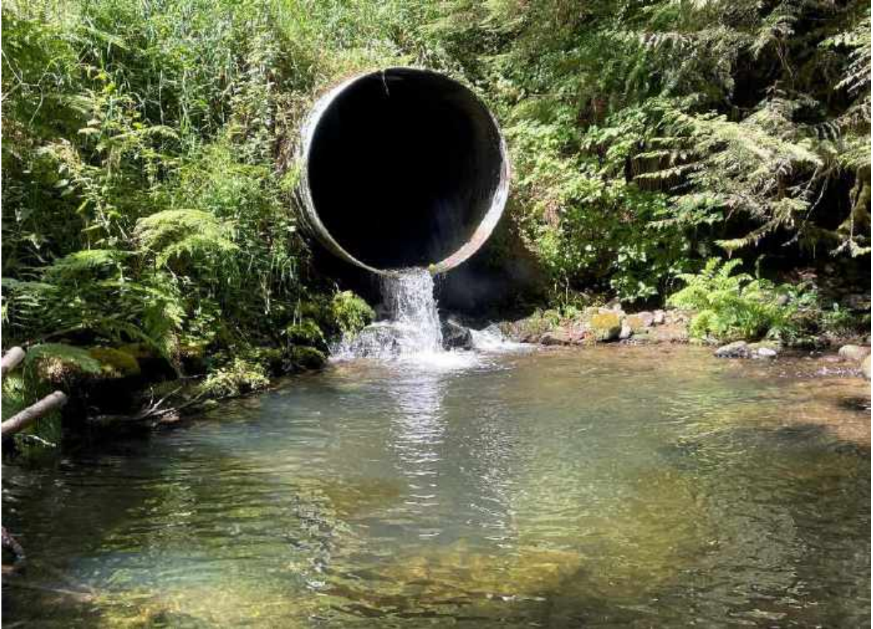
Photo 30: Campbell Creek perched culvert
